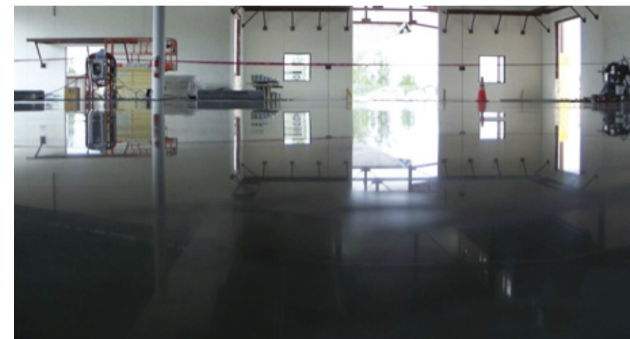
Attaining the desired level of shine in polished-concrete installations depends on the number of passes of the diamond disc grinder, as each step increasingly flattens the floor and enhances light reflectivity.
