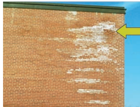
This photo shows an example of moisture leakage through a wall. The moisture picks up the salts from internal wall materials as it moves from inside the building to the outside. When the sun comes out, the salt solution dries, leaving a salt deposit, called efflorescence, on the surface. Efflorescence is a possible sign of a building-envelope problem.
