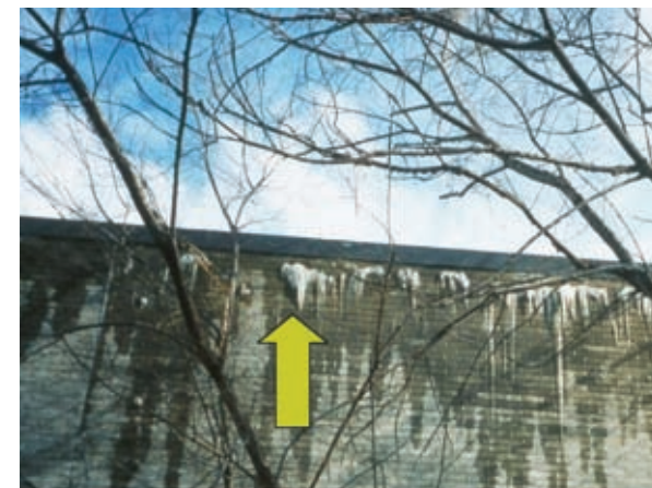
Here is another, perhaps more extreme example of moisture leakage. Enough moisture has leaked to form icicles on the exterior of the building.
